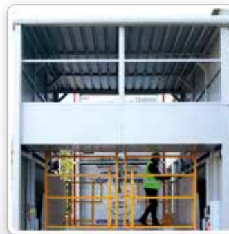
CLAD, ENCLOSED LOADHOUSE GIVES OPERATIVES A SHELTERED, WEATHERPROOF WORKING ENVIRONMENT
