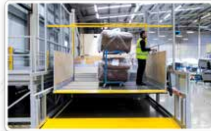
WAREHOUSE LIFT BETWEEN SPLIT LEVELS IN THE WAREHOUSE OR FACTORY
