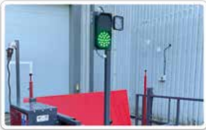
▲ LED Traffic Lights Interlocked to control panel
